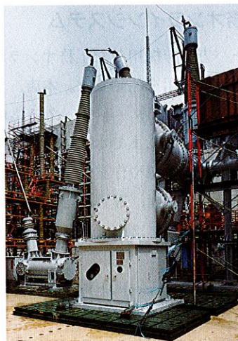
300 kV-63kV GIS 300 kV-63 kA gas-insulated switchgear
