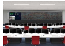
Central load-dispatching office system
