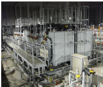
Multi-nuclide removal equipment
