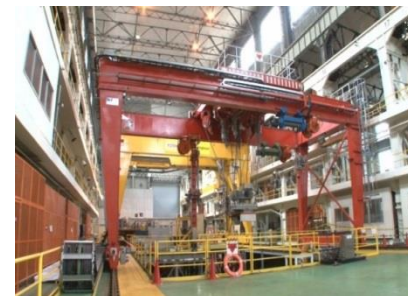
Fuel handling system
