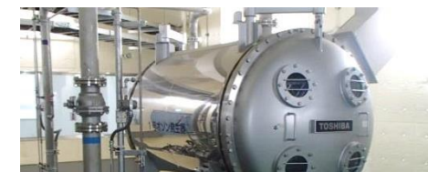
Kitachiba Water Supply Authority Advanced water treatment facility
