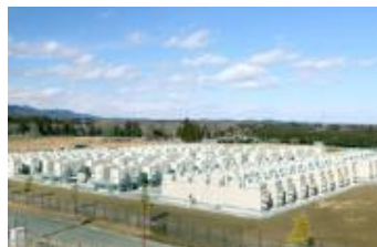
Tohoku Electric Power Minami Soma substation supply and demand balance improved by storage battery system
