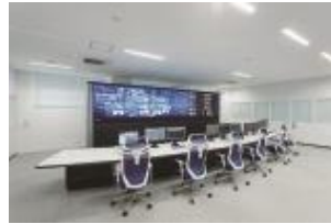
Monitoring control systems
