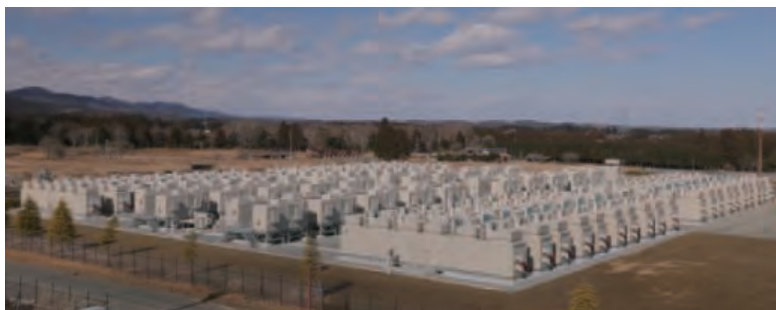
Toshiba's SCiB™ supports the battery energy storage system at Minami-Soma power transmission substation
