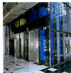
Advanced features guarantee unsurpassed comfort and reliability in Toshiba's ultra-high-speed elevators, like this model installed at Cosmotower in Osaka.
