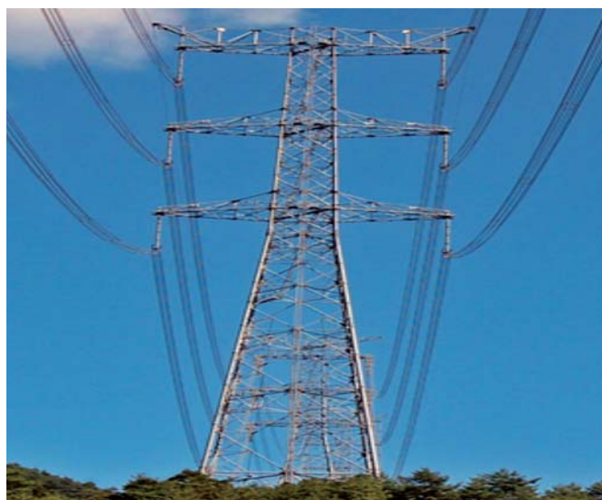
Transmission line for UHV (1,000kV) of TEPCO
