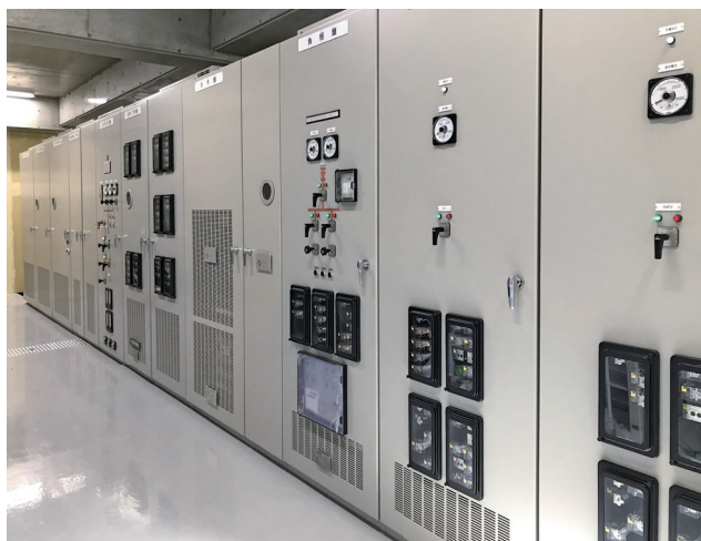
パッケージ型変電所 Package-type substation with integrated power receiver, transformer, main switchboard, and monitoring panel functions
