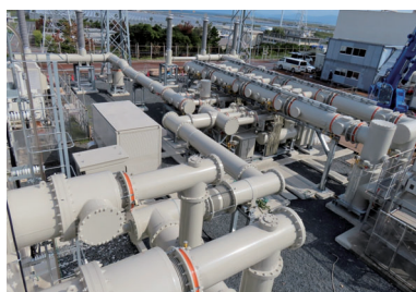
240 kV GIS 240 kV GIS installed at Kyushu Electric Power Transmission and Distribution Co., Inc. Wakamatsu Substation
