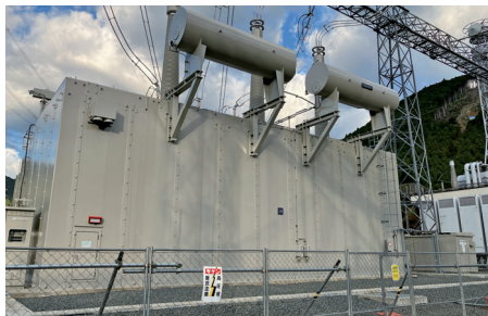
500 kV-1,500 MVA 変圧器 500 kV-1 500 MVA transformer installed at Chubu Electric Power Grid Co., Inc. Toei Substation
