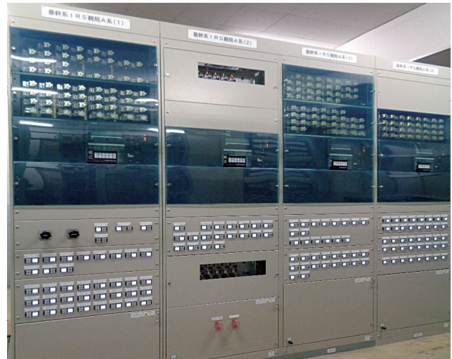
親局装置(デジタルリレー) Master station (digital protective relays)
