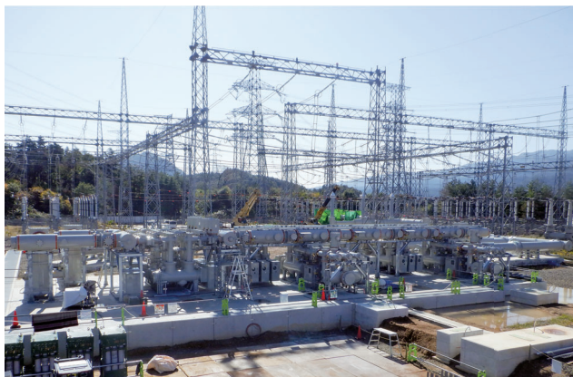
新形 300 kV GIS New 300 kV gas-insulated switchgear (GIS) installed at Echigo Switching Station
