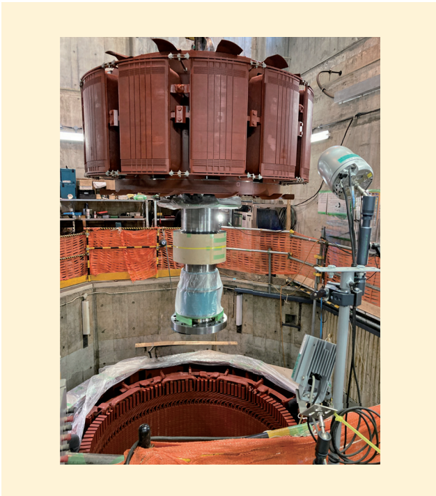
発電機の回転子つり込み Installation of generator rotor at Electric Power Development Co., Ltd. Ogamigo Hydropower Station
