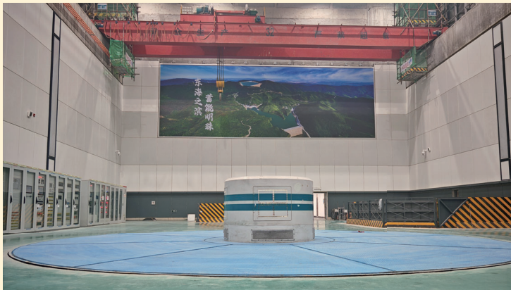
浙江寧海揚水発電所の全景 Ninghai Pumped-Storage Power Station, China
