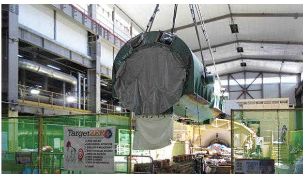
固定子コイル巻き替え後の旧発電機固定子のつり込み作業 Hoisting old generator stator onto foundation after stator coil rewinding at Calaca Power Station Unit 2, Philippines
