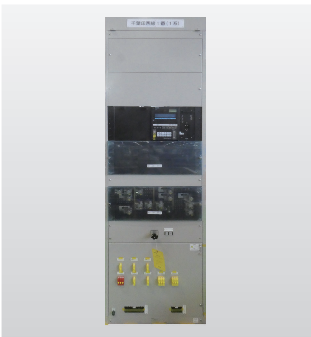
保護リレー装置 Protection relay equipment for Chiba-Inzai Substation of TEPCO Power Grid, Inc.
