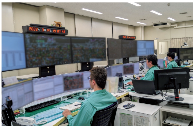
愛媛系制システム指令室 Control room at Ehime Grid Control Center of Shikoku Electric Power Transmission & Distribution Co., Inc.
