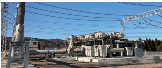
北陸電力送配電（株）加賀変電所 300 kV GIS 300 kV GIS for Hokuriku Electric Power Transmission & Distribution Company Kaga Substation
