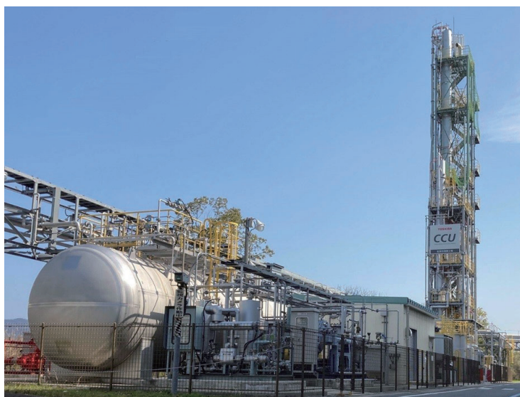
佐賀市清掃工場CO 2 分離回収設備 Carbon dioxide (CO 2 ) capture facility at Saga City waste incineration plant
