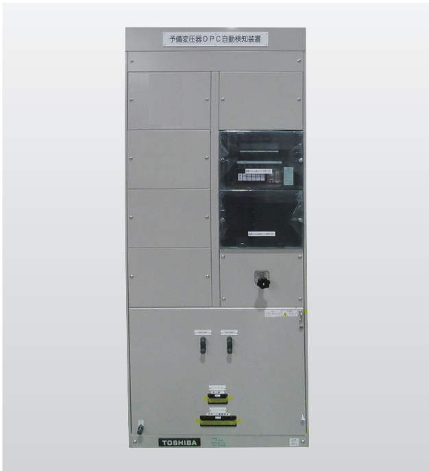
OPC自動検知装置 Automatic open-phase condition (OPC) detection device
