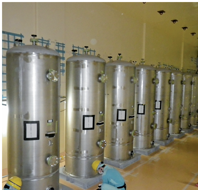
廃ガス貯留設備（工事完了後） Completed active vessel off-gas treatment units
