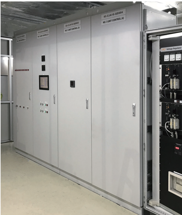
発電機制御盤 Control panel for Nam Ngum 2 Hydroelectric Power Station Unit 3, Laos
