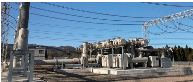
北陸電力送配電（株）加賀変電所 300 kV GIS 300 kV GIS for Hokuriku Electric Power Transmission & Distribution Company Kaga Substation
