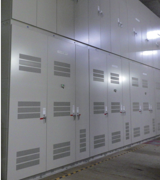
更新後の二次励磁装置用変換器 New power converter for secondary excitation device at Electric Power Development Co., Ltd. Okukiyotsu No. 2 Power Station
