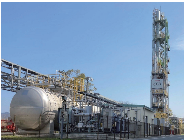
佐賀市清掃工場CO 2 分離回収設備 Carbon dioxide (CO 2 ) capture facility at Saga City waste incineration plant
