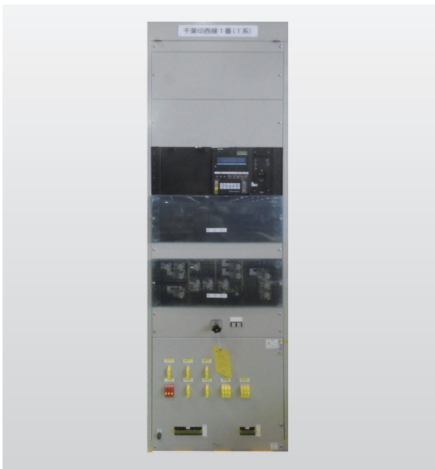
保護リレー装置 Protection relay equipment for Chiba-Inzai Substation of TEPCO Power Grid, Inc.
