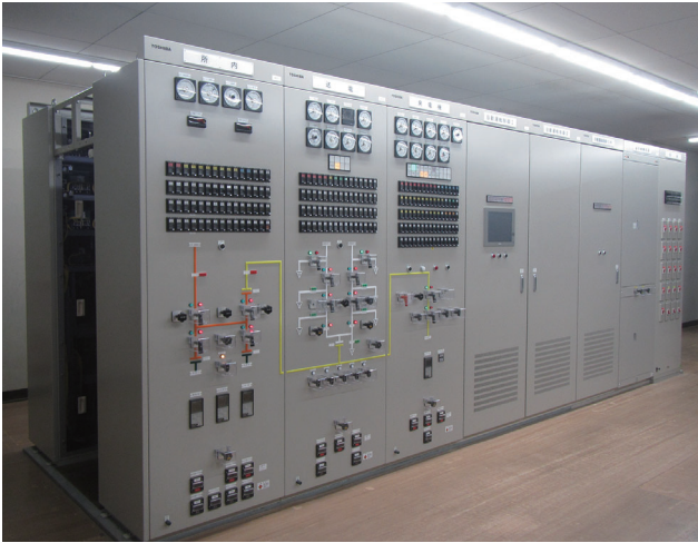
配電盤 Control panel for Hokuriku Electric Power Company Arimine Daiichi Power Station
