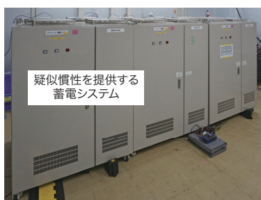
慣性力を提供するGrid forming inverterを検証する実証実験装置 Demonstration facility to verify grid-forming inverter with inertia-supported control technology
