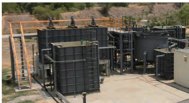
大容量高速沈殿槽の実証試験設備 Demonstration test facility for high-rate clarifier with larger capacity than that of existing products
