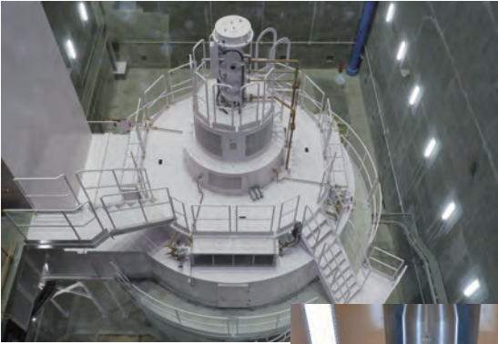
市房第一発電所の水車・発電機 Hydraulic turbine generator for Ichifusa No. 1 Hydroelectric Power Station of Kumamoto Pre- fectural Government
