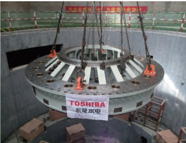
水車上カバーのつり込み Installation of turbine head cover at Jiangpinghe Hydropower Station, China
