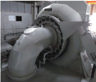
矢代川第一発電所の水力発電設備 Hydraulic equipment for Yashirogawa No. 1 Hydroelectric Power Station of Joetsu Energy Service Co., Ltd.
