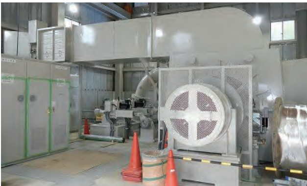
矢代川第二発電所の水力発電設備 Hydraulic equipment for Yashirogawa No. 2 Hydroelectric Power Station
