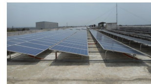
Solar panels installed on the rooftop of building in Unit-3
