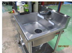
Automatic faucet and sink
