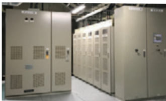
Traction energy storage system with SCiB™ for DC railway power supply systems (for Okinawa Urban Monorail, Inc.)
