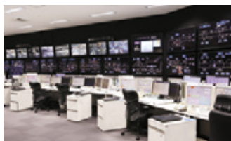
Traffic & information control system (for Tobu Railway Co., Ltd.)
