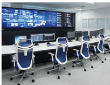
Monitoring and control system for water supply and sewage treatment plant
