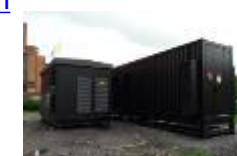
Helen OY (Finland) 1.2MW-0.6MWh
