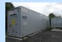
University of Sheffield (UK) 2MW-1MWh
