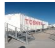
TERNA Virtual Storage Plant (Italy) 1MW-1MWh
