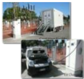
ACEA Smart Grid Project (Italy) 10kW-45kWh
