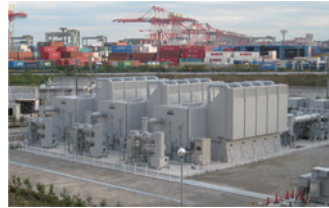
275kV-300MVAガス絶縁変圧器 275kV-300MVA Gas Insulated Transformer
